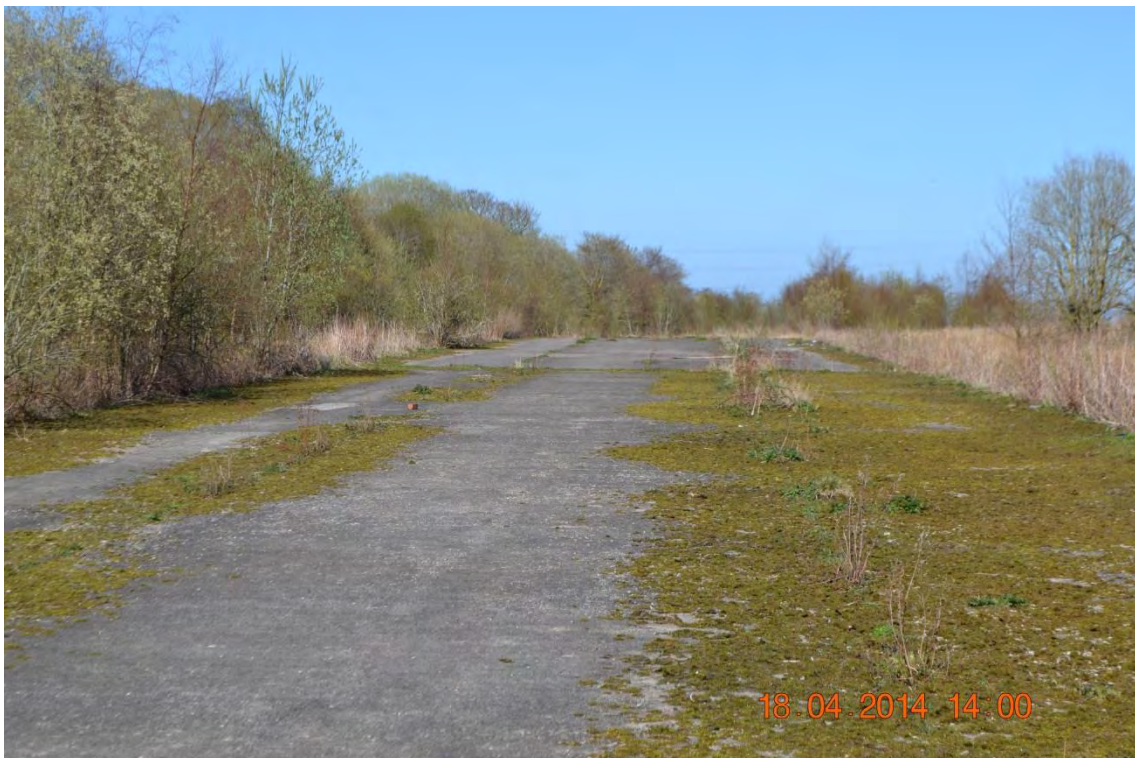
Photo 6 – Poultry site, remaining hatchery foundations (100yrs plus design life), strewn with waste.
