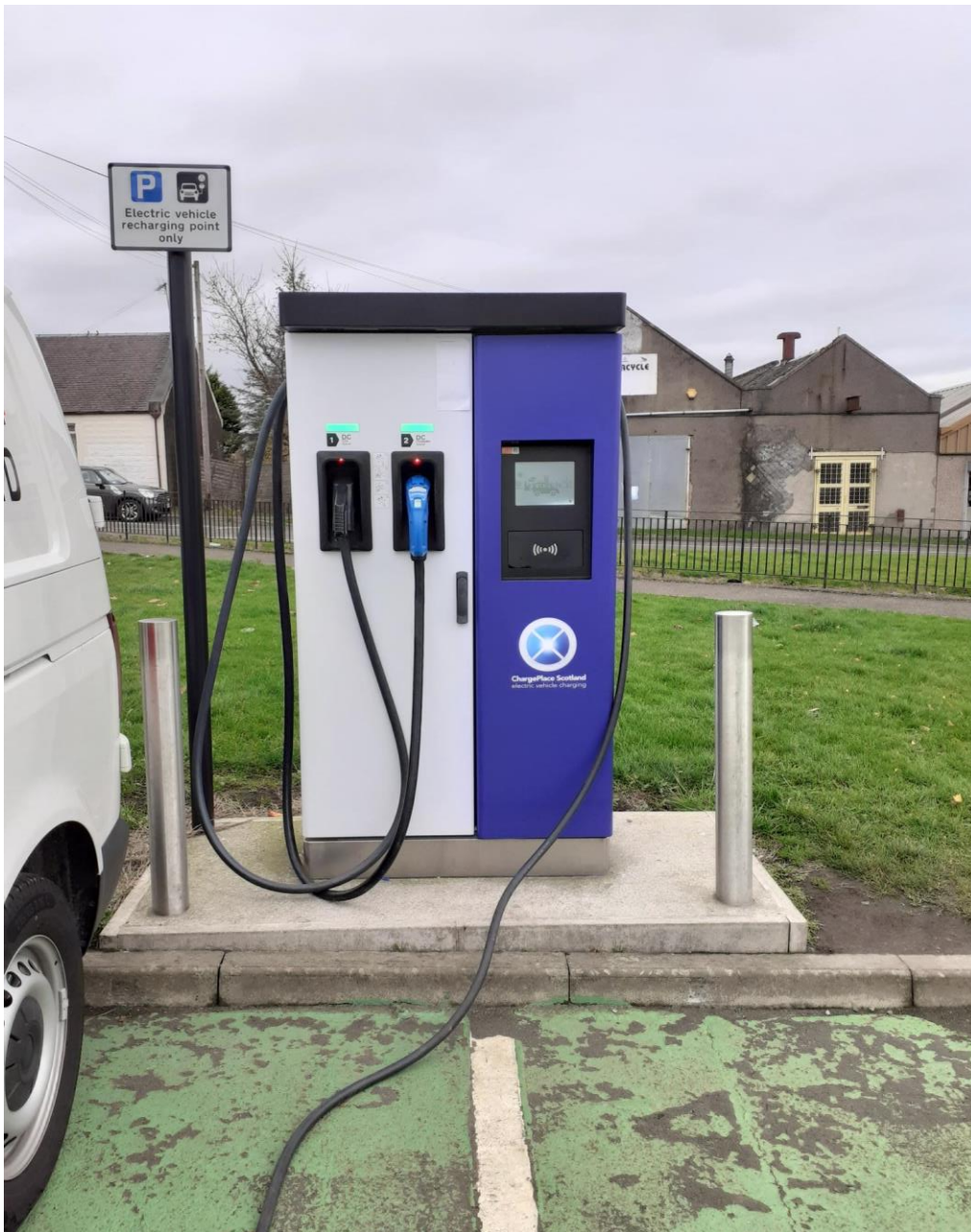
New EV charging point with public access installed at the Strathbrock Centre, Broxburn
