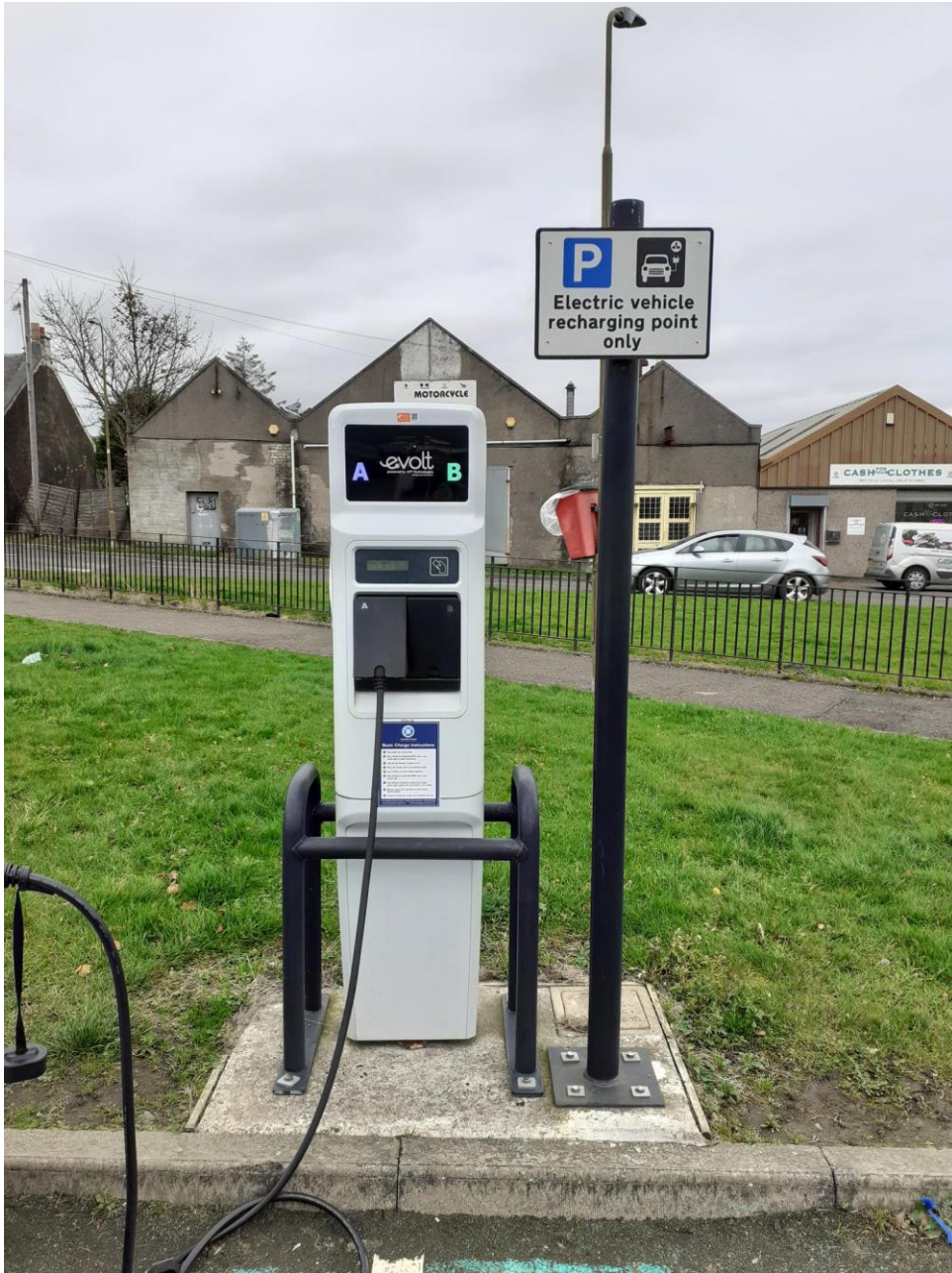
New EV charging point with public access installed at the Strathbrock Centre, Broxburn
