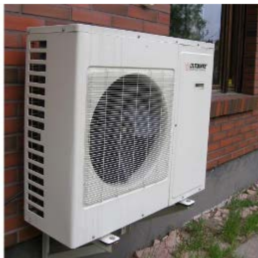
Figure 8: An Air Source Heat Pump
