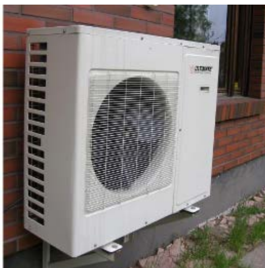
Figure 8: An Air Source Heat Pump
