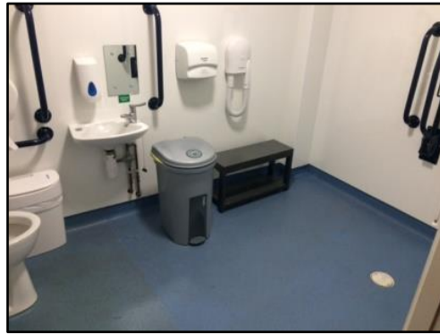
Disabled shower room – camping block
