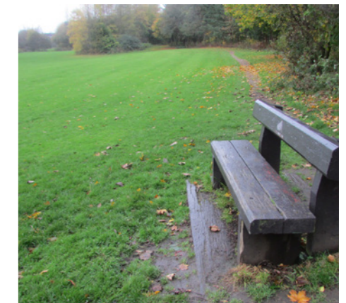
timber seating at the end of its life needing to be replaced
