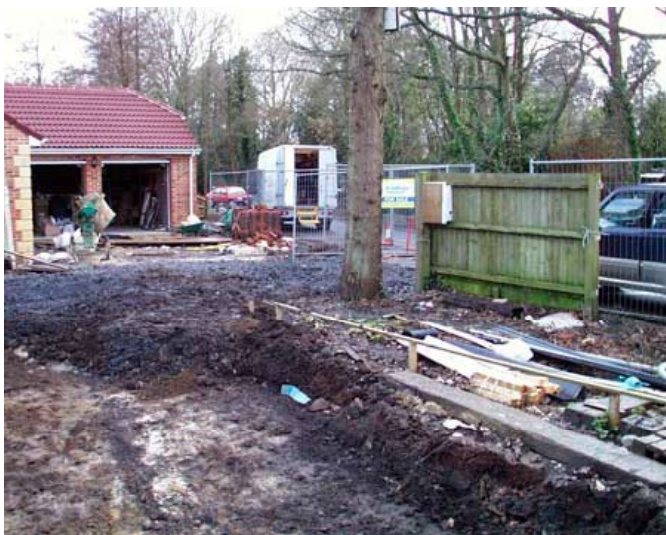
This tree has suffered both root damage and compaction damage due to vehicle movements and storage of materials. This tree is unlikely to survive.
