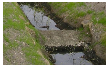
Check Dam to control flow velocity
