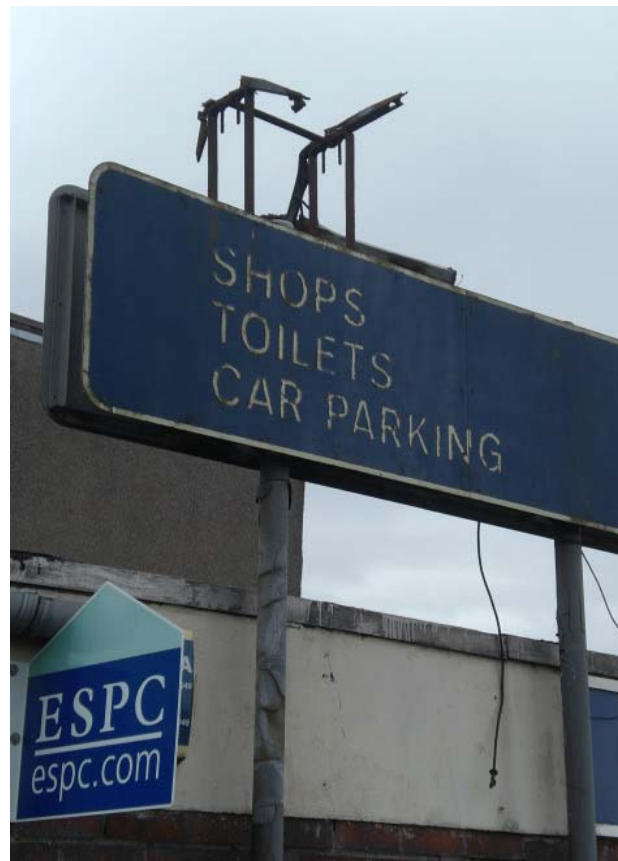
Example of poor quality signage in the town centre
