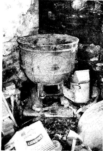
22. Quarter Farm: boiler.
