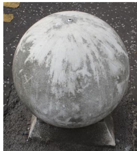
Large, cylindrical concrete bollards around West Port are a potential trip hazard and contrast with black cast-iron street furniture located elsewhere along the High Street.
