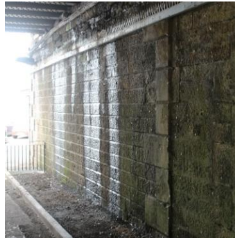
Poorly lit, unsightly and uninspiring underpass leading to Station Road immediately adjacent to train station exit.
