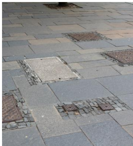
Left: Poor quality implementation and attention to detail detracts from quality of materials and leads to potential trip hazards
