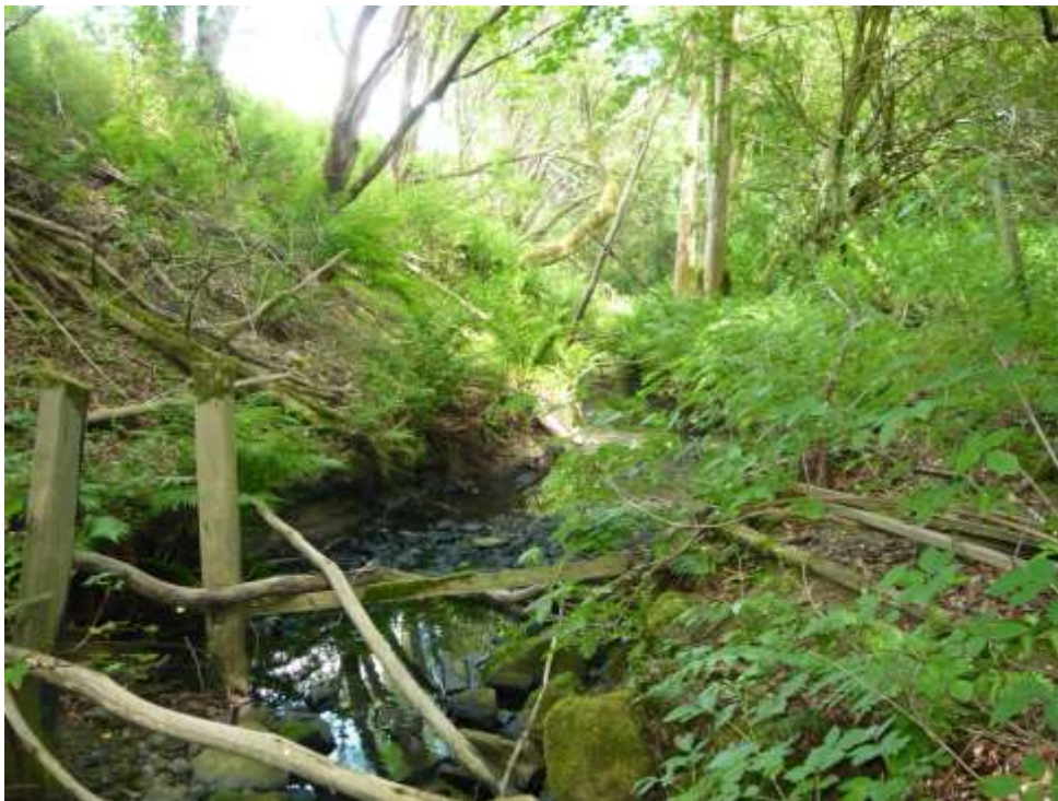
Plate 2: View of unnamed stream downstream of site from Murieston Road culvert
