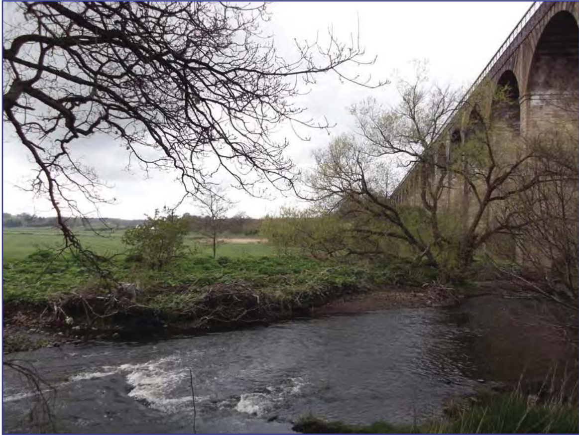
Plate 3: Edinburgh to Glasgow Railway Viaduct, River Avon (Avon Viaduct) (Site 16) from east
